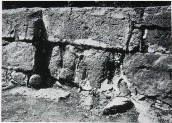
FIG. 120 - PALACE OF KATO ZAKRO SET-BACK IN WESTERN SIDE OF CENTRAL COURT - NOTE PLASTERING
