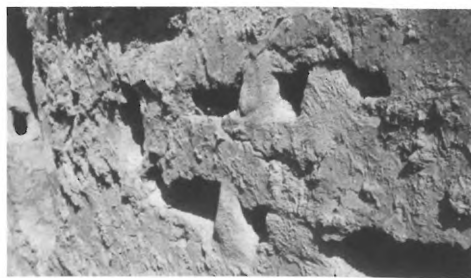
64 - VASILIKI - PARTIALLY RESTORED WALL, SHOWING HARD PLASTER FACING AND CAVITIES CAUSED BY THE DISINTEGRATION OF WOODEN BEAMS (LOOKING WEST).
