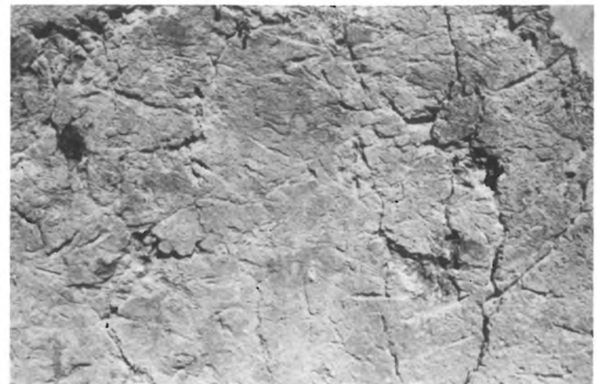
253 – TYLISSOS - HOUSE C - COARSE MUD PLASTER WITH IMPRESSIONS OF STRAW BINDER IN CORRIDOR B.
