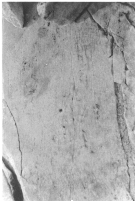
b. Bottom of drum D10 224J with incised guide lines for the placement of an empolion
