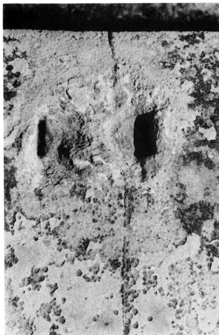
FIG. 11. Calcined line from roof leak at joint of flank sima
