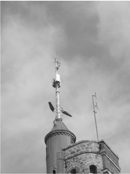
Fig. 31.19. Practical example of a translator or gap-filler site; the 2 (log periodic) receiving antennas are located in the lower part of the extended pinnacle of the tower, the 3 transmitting antennas (8-element bays) are located in its upper part
