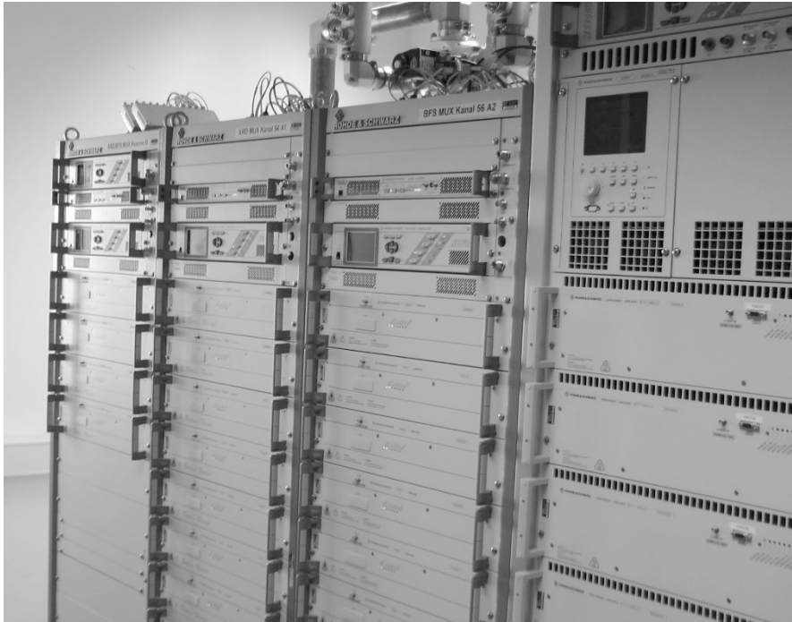
Fig. 46.5. DVB-T transmitter racks, transmitter station Wendelstein, Bayerischer Rundfunk
