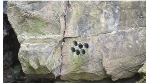
Moel Hiraddug Quarries, Wales, highly visible coring damage Photo. Raymond Roberts, Countryside Council for Wales
