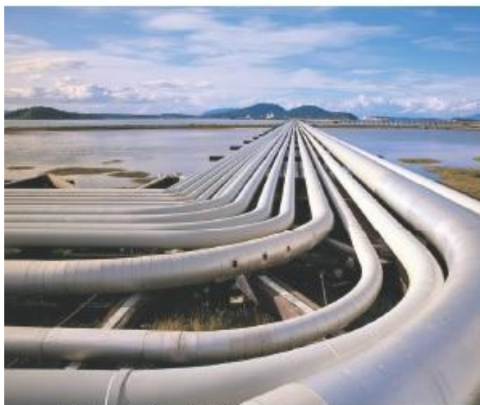
A petroleum pipeline at Anacortes, Washington.
